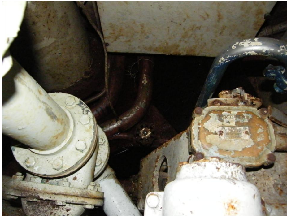
Standing oil in Pumproom.
