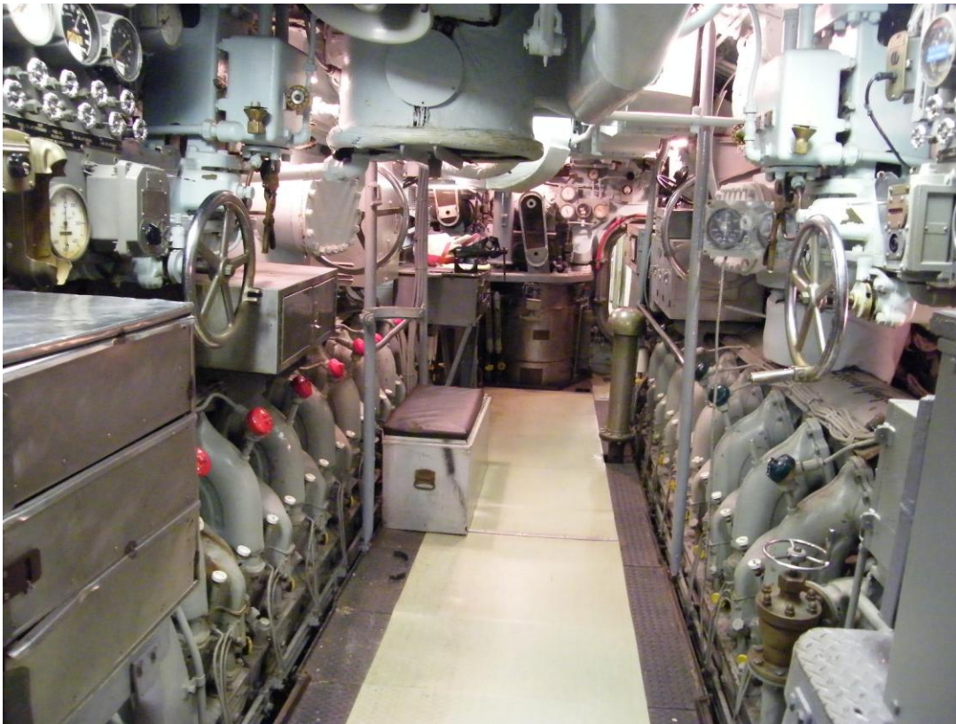
Forward Engine room, looking aft..
