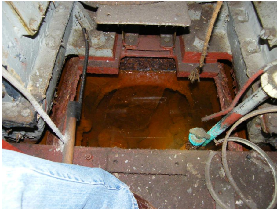
Standing water on centerline bilge of lower motor room.
