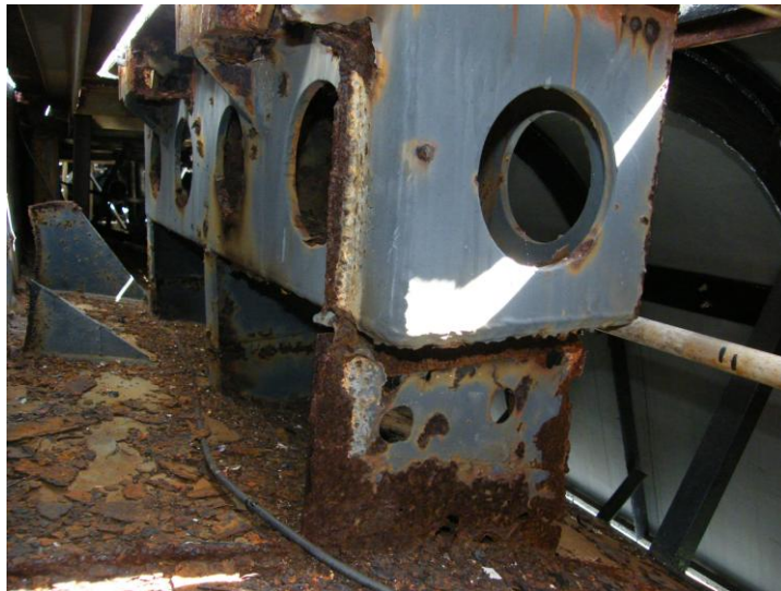
Wasted mooring cleat foundation, typical of superstructure deck material condition.
