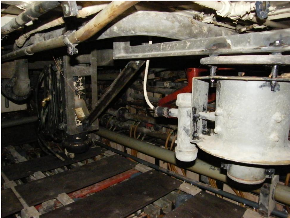
Forward Battery Room, looking aft to port.
