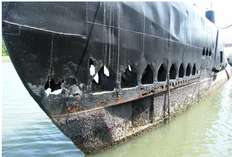
Overall view of port bow of CLAMAGORE, showing wasted plating for superstructure fairing.
