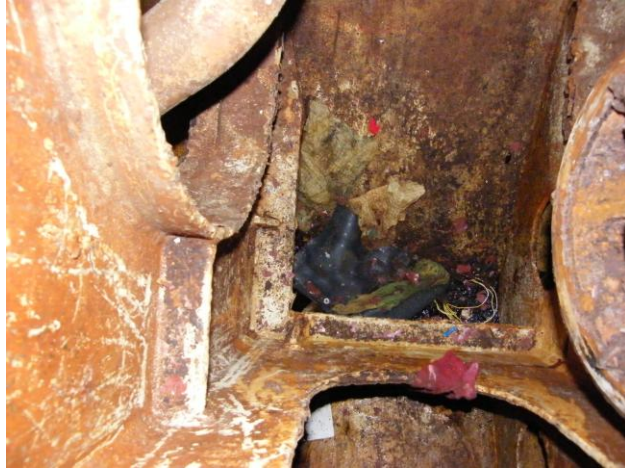
Interior of Forward Trim Tank.
