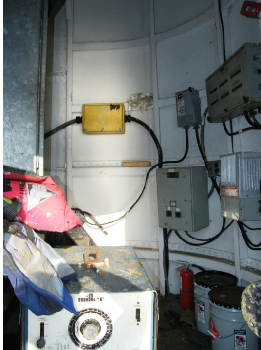
Maindeck access to sail with assorted shore power boxes and transformers.
