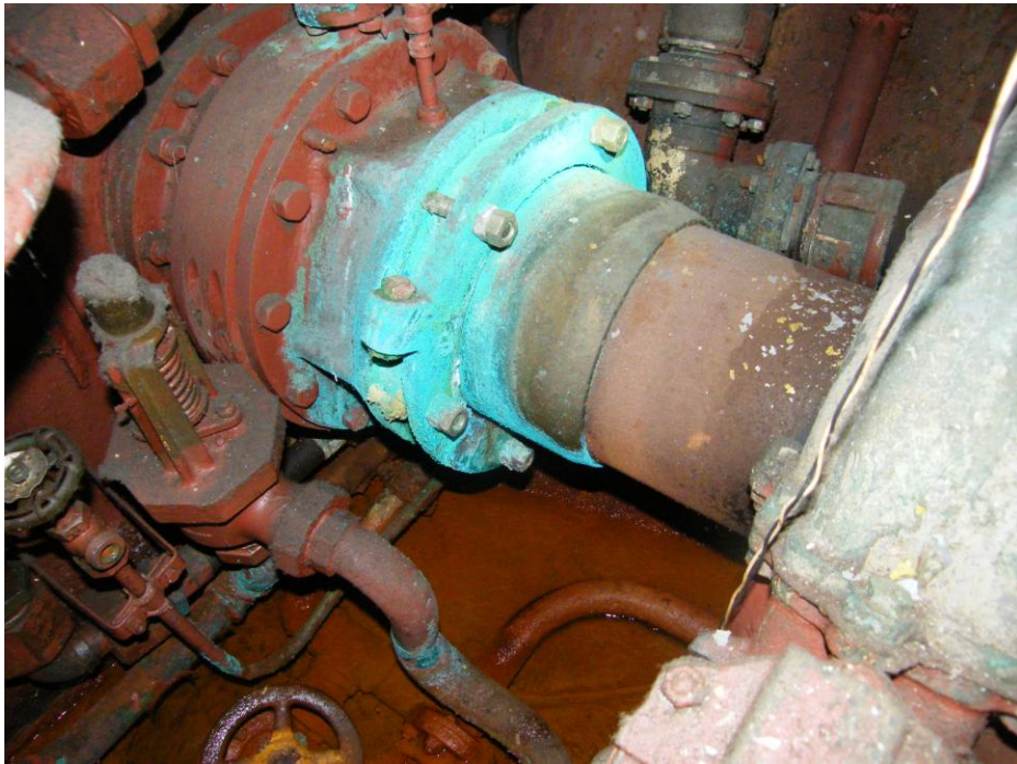
Port shaft packing gland in lower aft motor room. Showing weeping packing gland and standing water in bilges.
