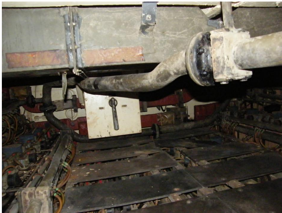
After Battery Room, looking aft.
