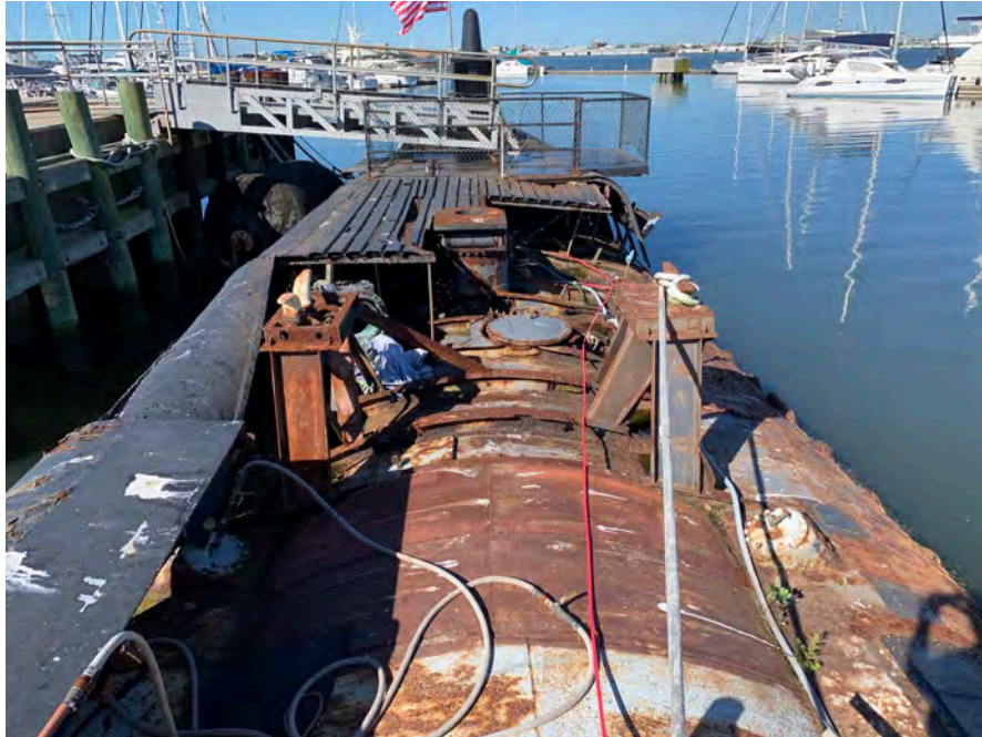
Superstructure deck atop pressure hull. This area requires total rebuilding throughout its length.
